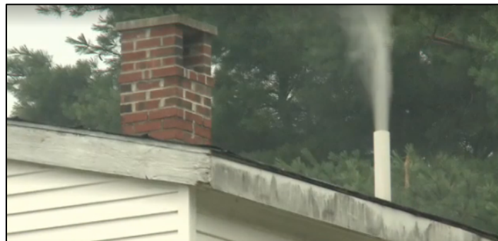
Smoke exiting through a plumbing roof vent is normal and expected
